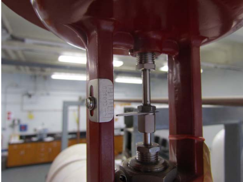
Pneumatic Valve Position
