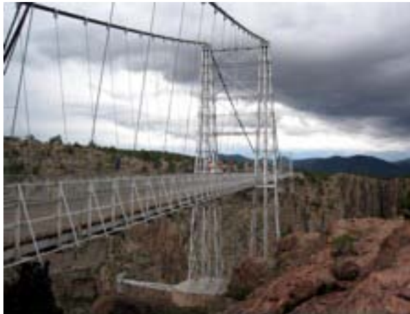
The Royal Gorge Bridge, one of the highest suspension bridges in the world
