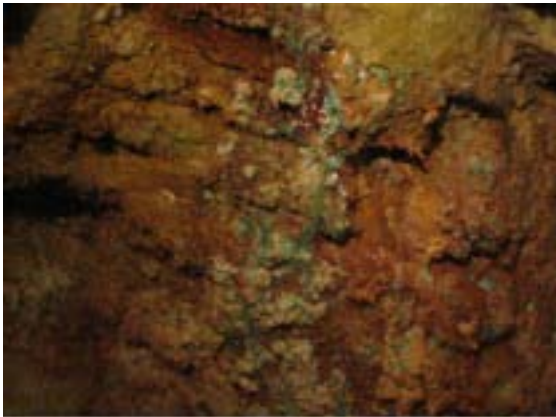
Mineral accumulations of copper, sulfur, and iron oxide line walls for portions of the mine
