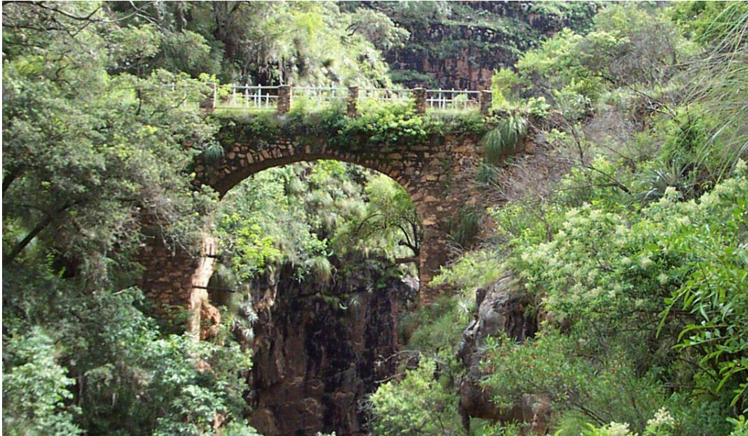
Figure 4.9: El Puente de los Libertadores , called so because Simon Bolivar passed across this bridge on his travels to the cities of Sucre and Potosi Photo courtesy Brad David Kennedy
