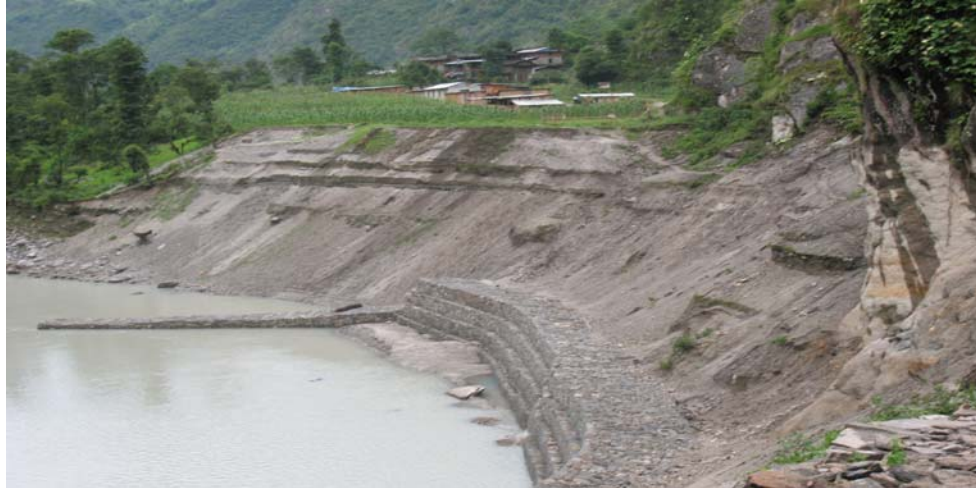
Figure 3-4. Gabion wall erected as part of mitigation efforts at Gongar (Photo by author).
