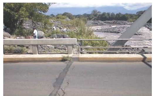
Photo 4.2 Cracks in the pavement of the bridge
