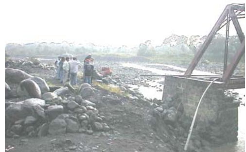
Photo 4.1 Destruction of Railroad Bridge over the Samala
