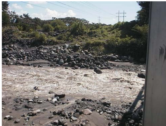
Photo 5.3 Sector of dike destroyed in 1988
